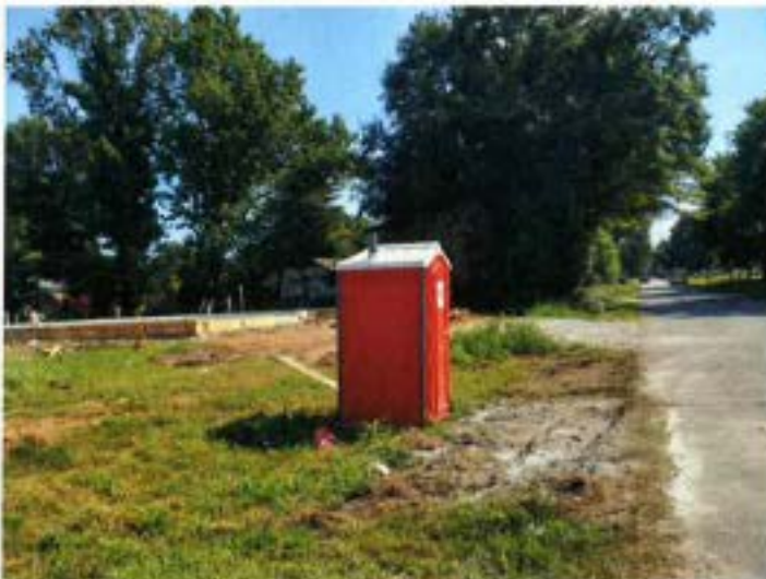
Subject Property where the proposed accessory building and single-family home are under construction.
